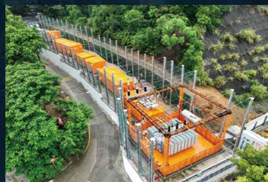
Substation load transition
