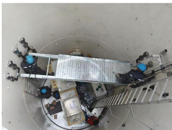
▲ upgrade from small to large turbines “以大代小”
