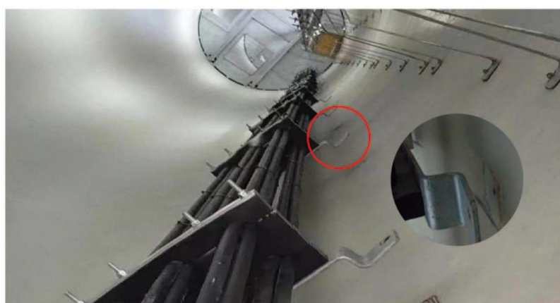
Failed shoot nail mounting system 射钉脱落实景图
