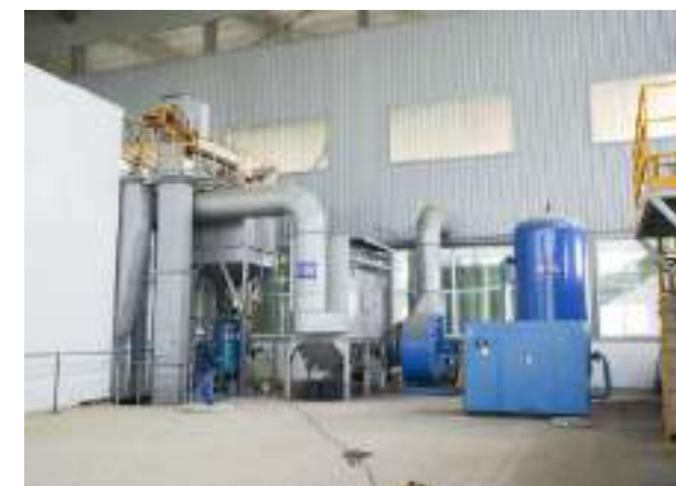
VOCs Waste Gas Treatment System
