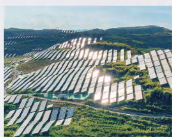
MOUNTAINOUS PHOTOVOLTAIC POWER STATION
