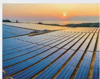
PLAIN PHOTOVOLTAIC POWER STATION
