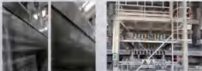
COMPARISON PICTURES OF THE INSIDE OF THE MOLD BEFORE AND AFTER THE OPERATION
