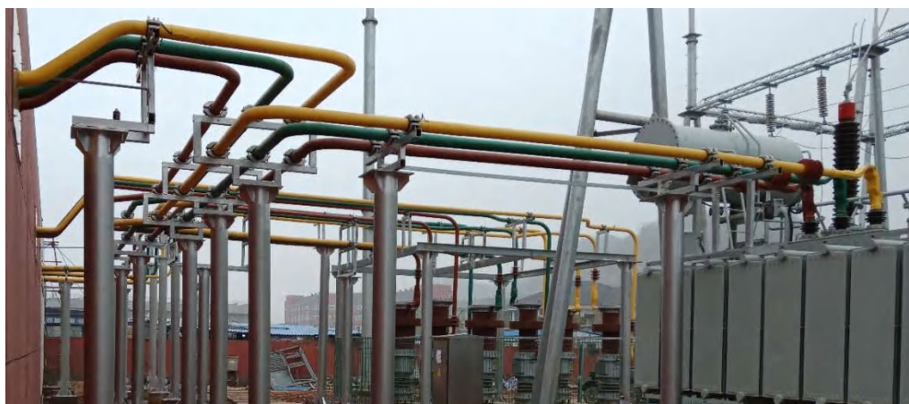
12kV/4000A Waste-heat Power Generation
