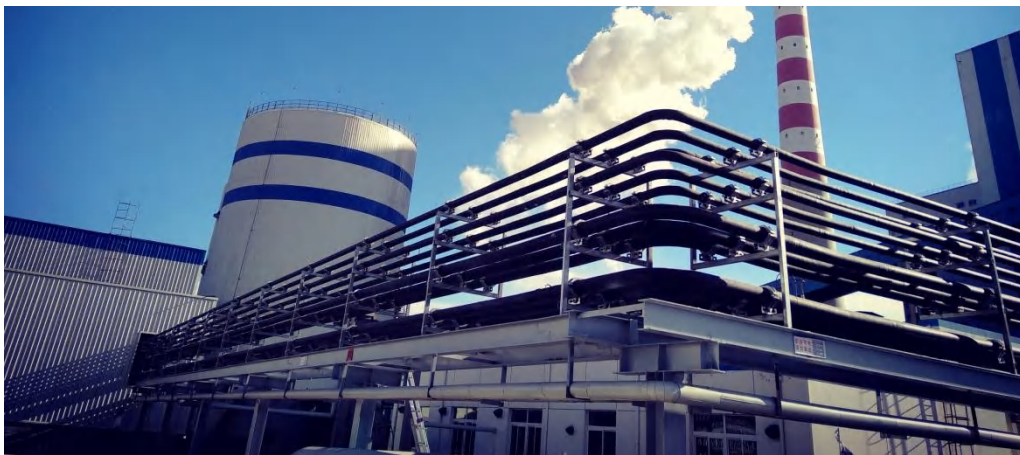
12kV/6300A Peak-shaving & Energy Storage
