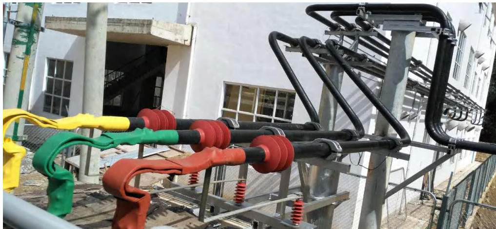
12kV/3150A Hydropower Generation
