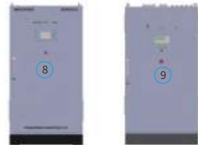
Figure 2 Inverter and Controller
