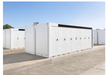
Energy storage system
